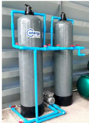
H 2 S Cleaning Tanks
